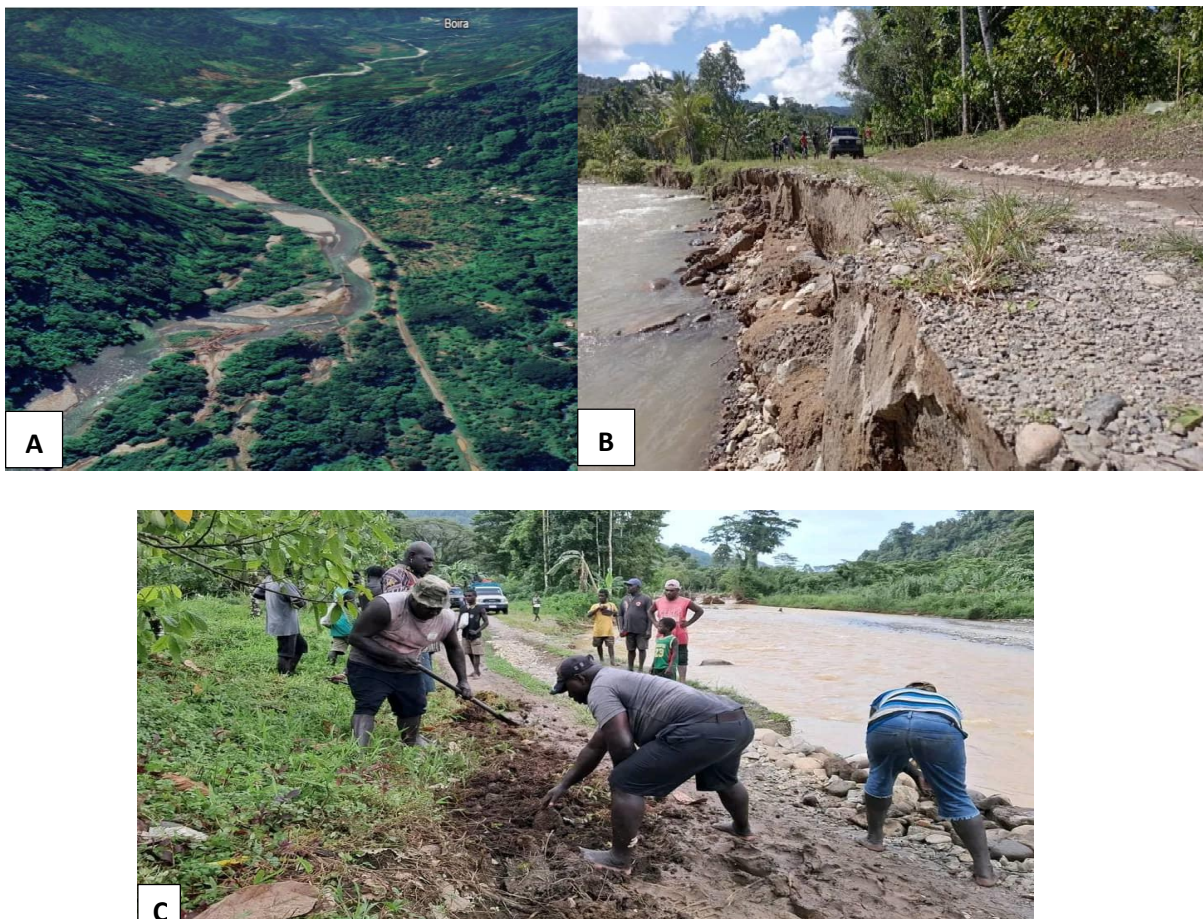
Figure 4. a) Ariel View of disrupted water flow pattern; b) Road affected due to water flow disturbance; c) Road affected due to sedimentation
